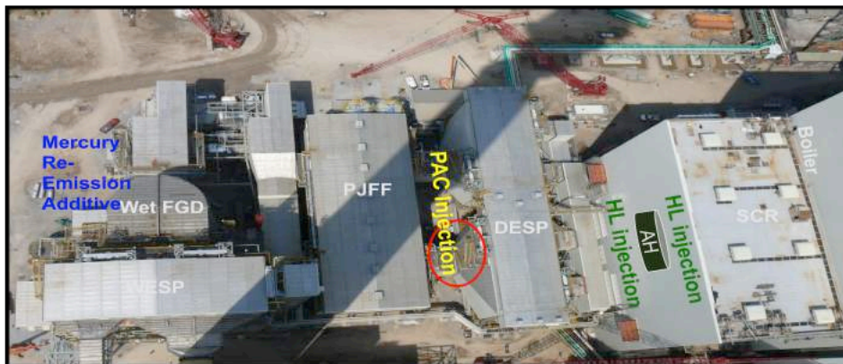
Figure 1 – Trimble County 2 AQCS and HLIS
