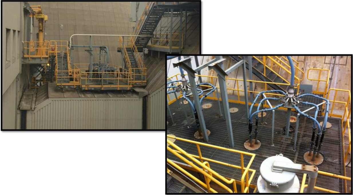
Figure 5 – ACI Injection Inlet – Analyzer Test Ports
