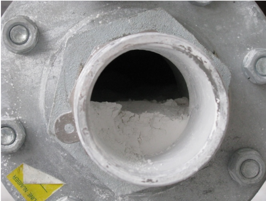
Figure 8 - Outlet of the Transition Chute below the Feeder after 38 days of operation
